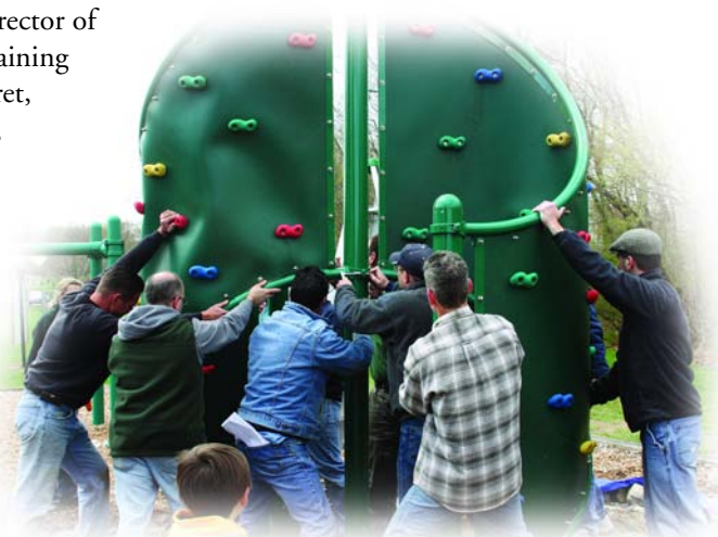
Parent volunteers and Laborer representatives working hard to ensure equipment is installed properly.
